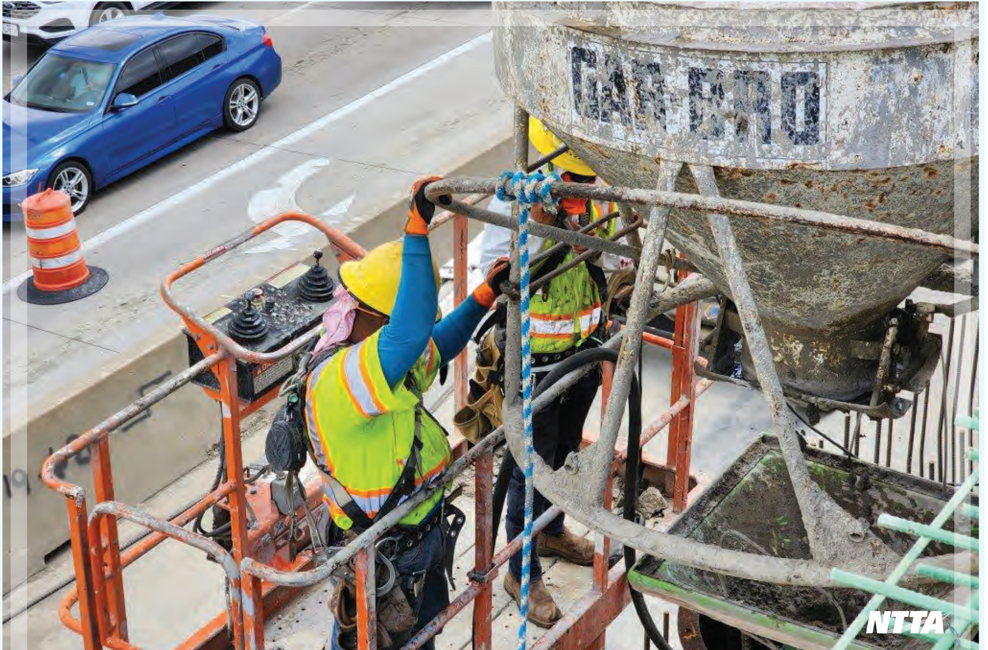
Pouring concrete for wall on Dallas North Tollway widening project in Frisco
