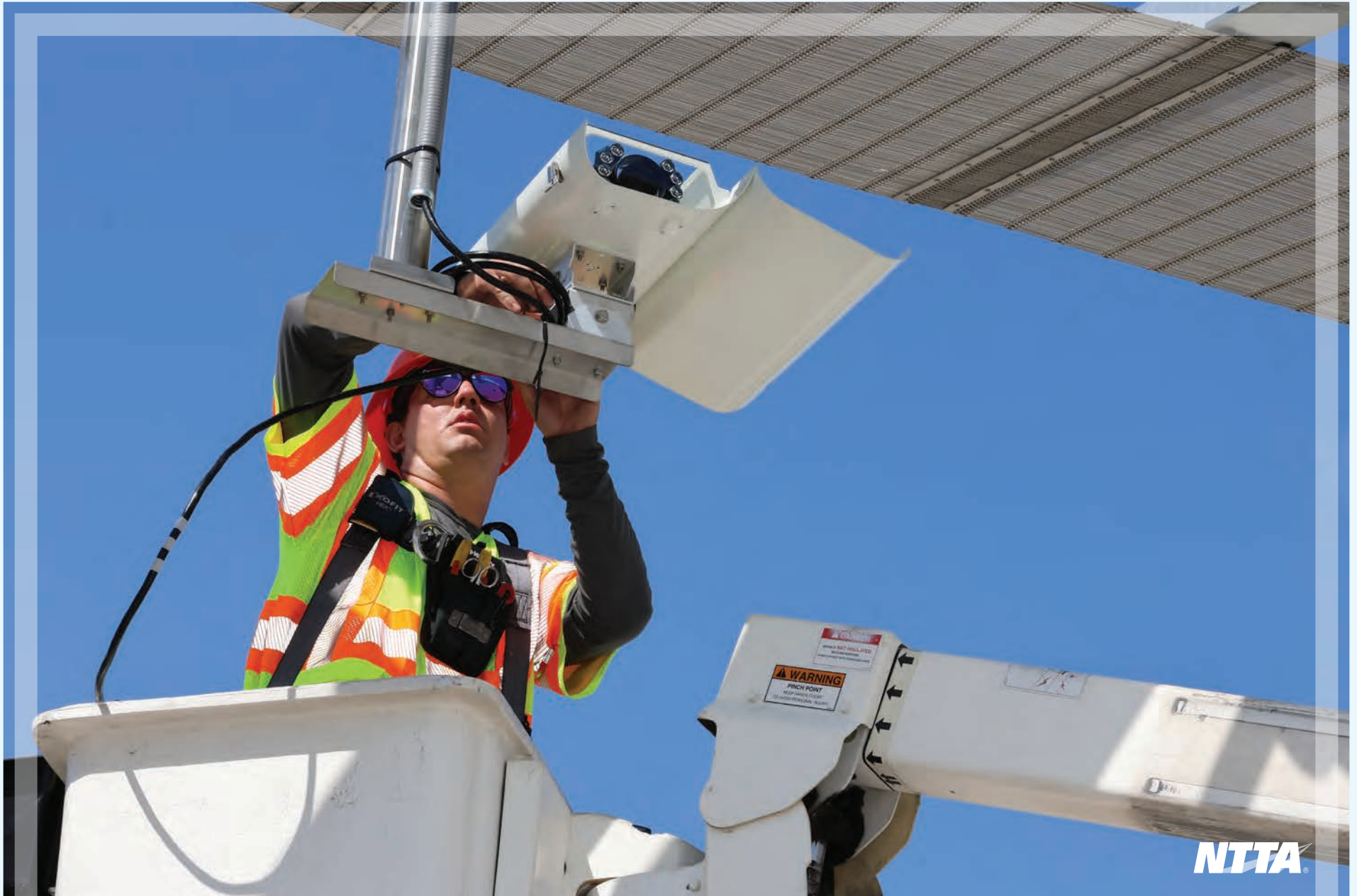
Roadway Information Technology installing new cameras on Dallas North Tollway in Frisco
