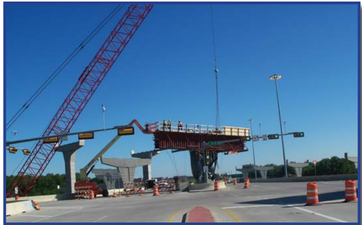
PGBT Western Extension construction crews set formwork for a bridge support at I-20.
