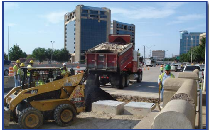
Crews working on the all-ETC (cashless tolling) project place asphalt under concrete paving at the DNT's Main Lane Gantry 2.
