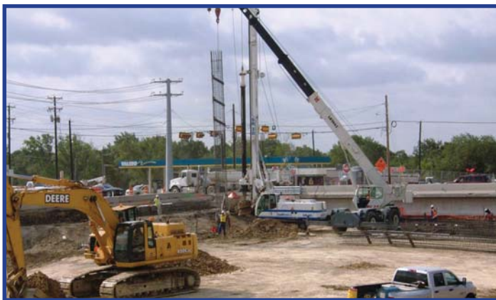
On the PGBT Eastern Extension project, crews place reinforcing steel for the SH 66 bridge support foundation.
