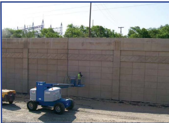
Crews finish a retaining wall in Section 2C of the CTP project.
